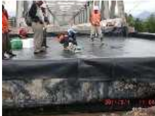
Field seams of geomembrane by hot shoe welding tool (Km 82+600 – Section 4) 01 Jun 2011
