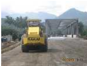
Compacting selected embankment capping layer near Lambeso north abutment (Km 82+700 – Section 4) - 09 Jun 2011
